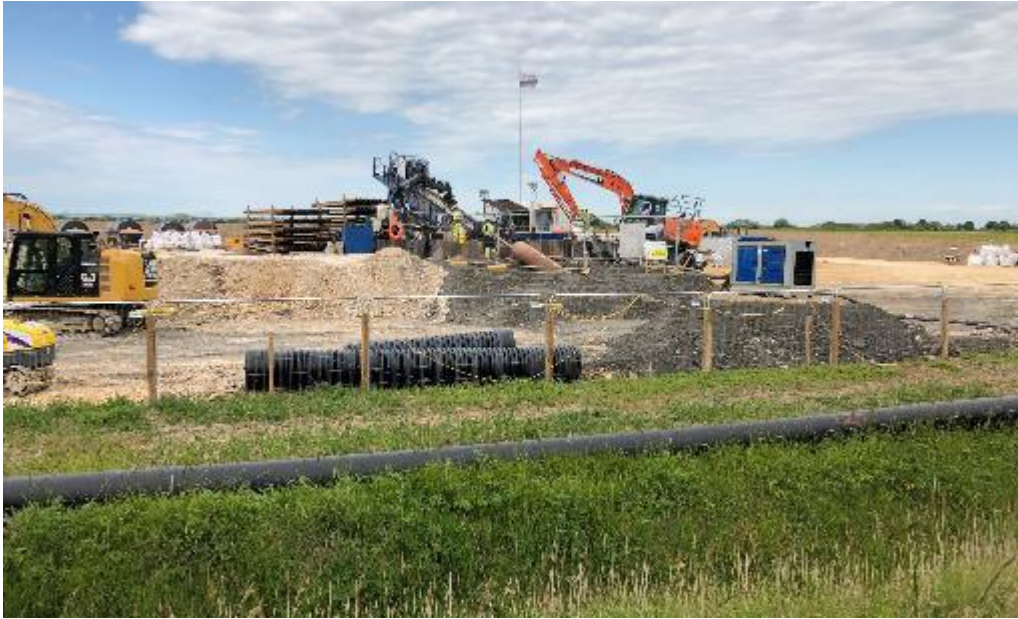
Plate 2.9 Example of a horizontal direction drill rig at landfall – the cable duct is closest in the foreground (image courtesy of RWE Renewables)
