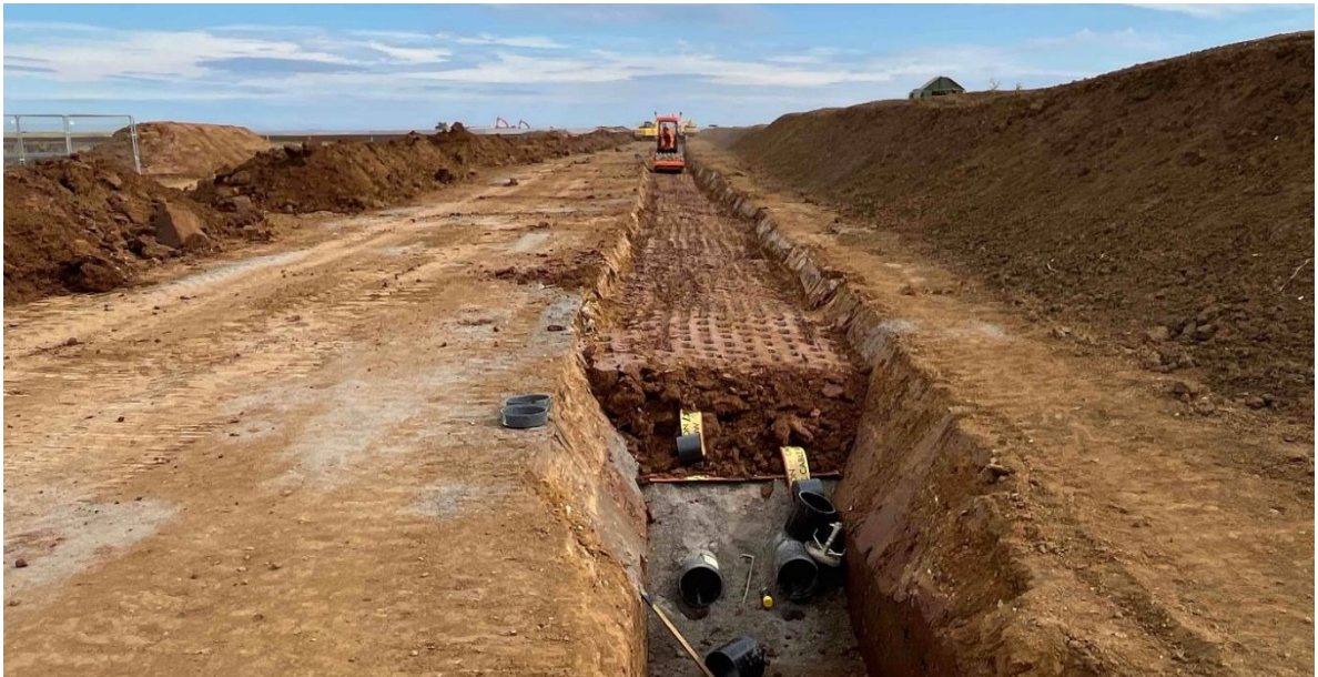
Plate 2.10 Example of a cable trench, once cable ducts have been installed and trench has been backfilled (image courtesy of RWE Renewables)
