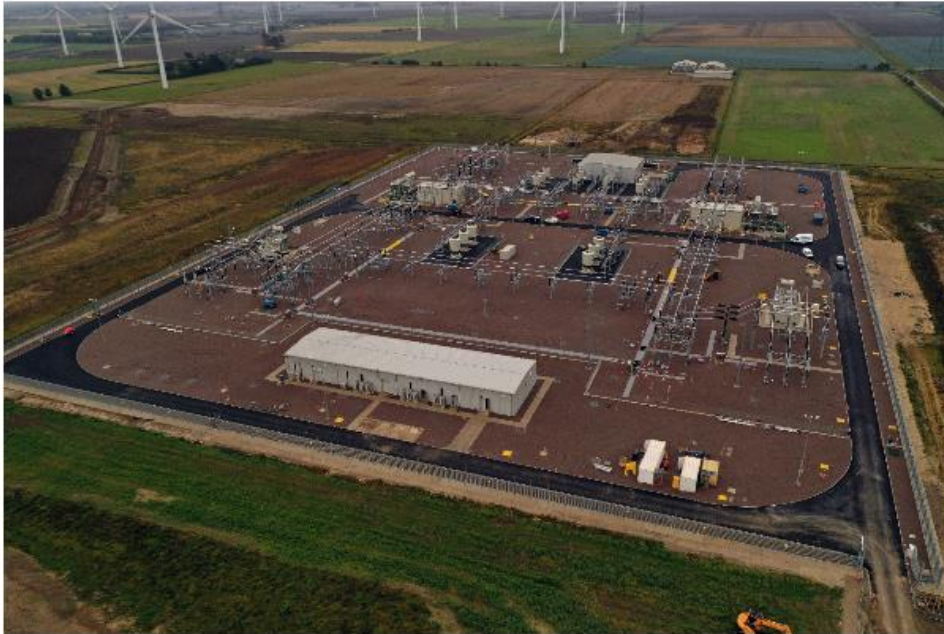
Plate 2.11 Example of an onshore substation (image courtesy of RWE Renewables)
