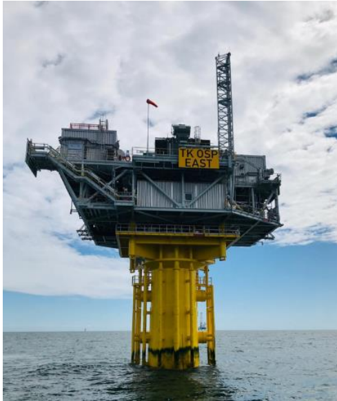
Plate 2.6 Example offshore substation platform (image courtesy of RWE)
